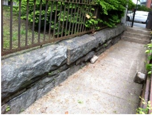
Wall with fallen/shifted stones – May 2015
